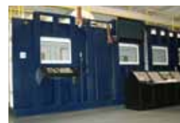
COMPUTER CONTROL AND MONITORING STATION
